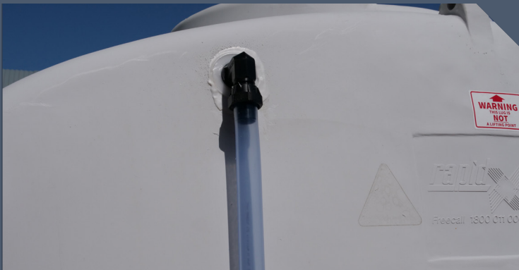
Sight Glass Water level sight glass.
